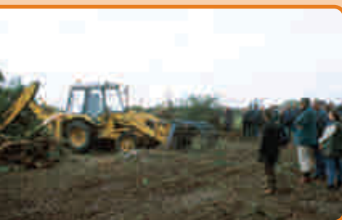
Contractor Gerald Sercombe, who's based at Slindon, demonstrates some heavy duty scrub-removing equipment.
